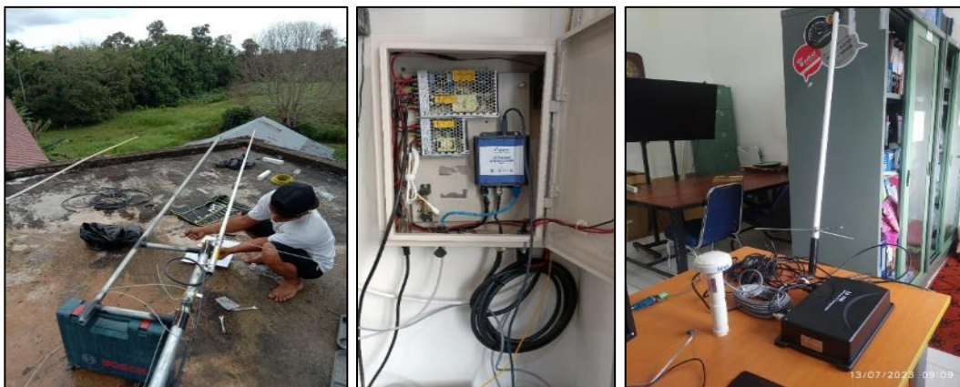
Figure 3. AIS Antenna Installation (Left), RBS Installation at Polbeng AIS Research Lab (Center), AIS Class B Device (Right)
