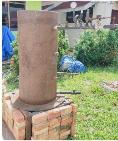
Figure 1, Boilerses vertical fire tube
