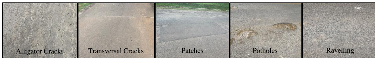
FIGURE 1. Type of Road Damage
